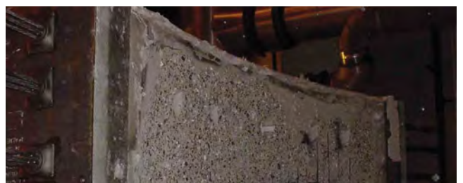
Exposed side of a tunnel segment after a fire resistance test. Spalling of concrete uncovered the reinforcement inside the concrete.
